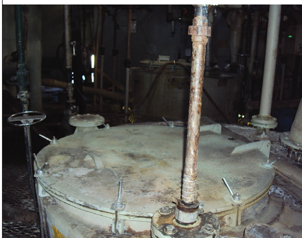
FIGURE 17 Processing equipment lacking maintenance
