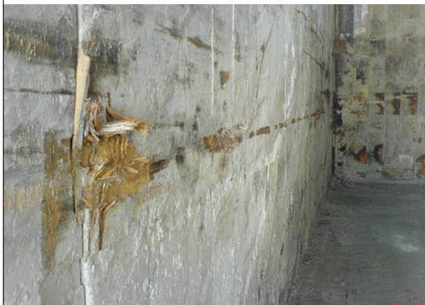
FIGURE 23 Bad bulk storage conditions
